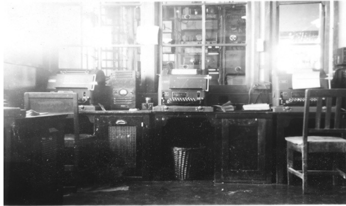
The landline teleprinter room in the late 1940s with the NZPO simolex line on the left, Navy Office inward in the centre and Navy Office outgoing on the right
